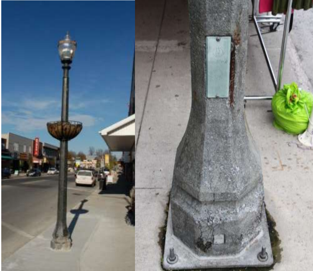
Figure 21. Existing StressCrete light pole in Listowel. Damage was observed on some poles.
